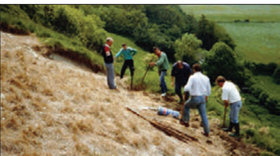
Fig 12. Restoration works about to start, the hill figure's chalk surface covered in growth. Metal stakes and a roll of chicken wire lay on the horse, ready to instal.
