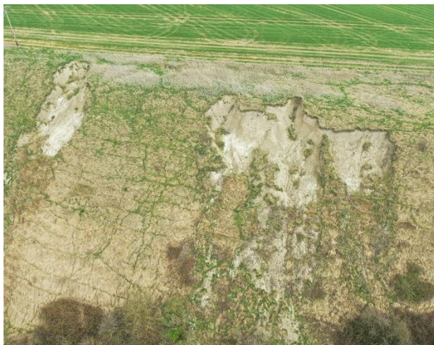
Figure 4: December 2023 landslips to the south-west of the white horse
